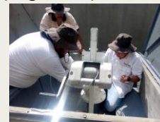
Figure 4. Upgrade PCRV Seismic Auxiliary Station (November, 2023).
