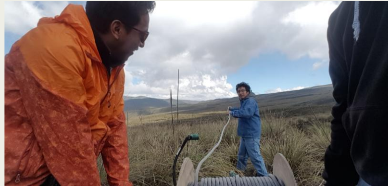
Figure 5. Prototype installation at remote location.
