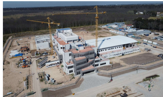
Panoramic view of RA 10 reactor. October 2023
