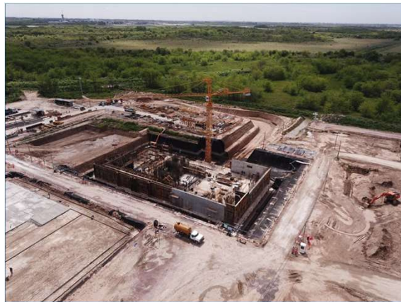
FQ 2018. Auxiliary building excavation finished. Reactor Building construction advanced. Neutron Beam Building started
