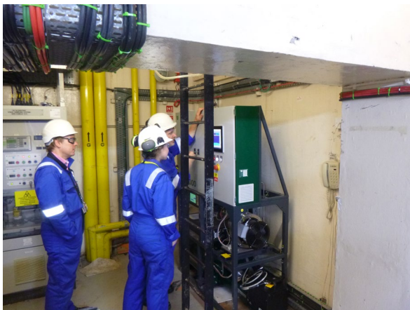
STAX system installed at the R6 tower in Hartlepool Power Station on the main blowdown route
