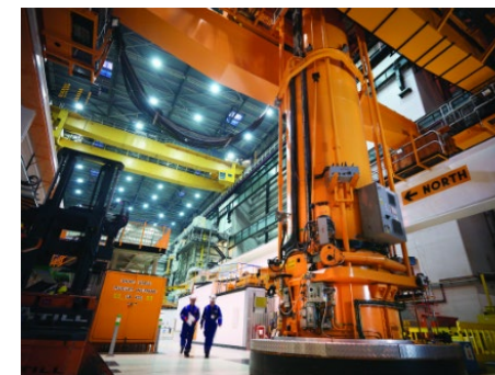
The Hartlepool power station fuelling machine
