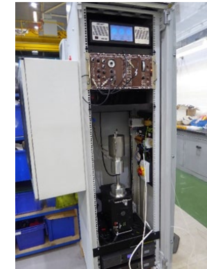
Gaseous Activity Monitoring (GAM) system at Hartlepool power station
