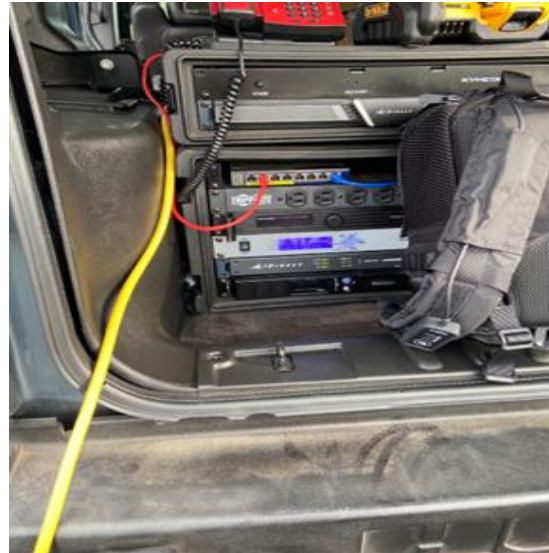
Mobile LEO equipment and networking equipment
