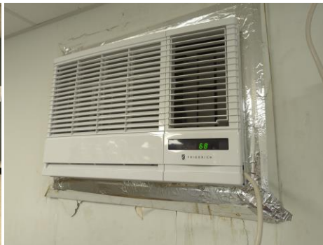
HVAC at GBP66
